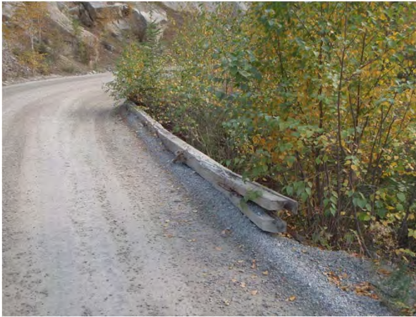
Figure 1-7: Left end approach, note condition of fender and overgrown vegetation.
