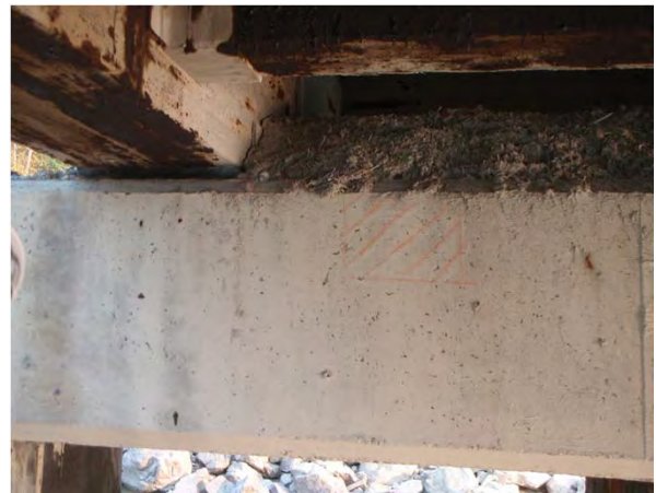
Figure 1-18: Pier 1 cap delamination.
